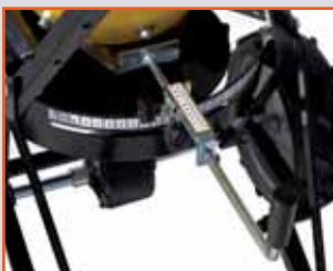
Gate opening control
